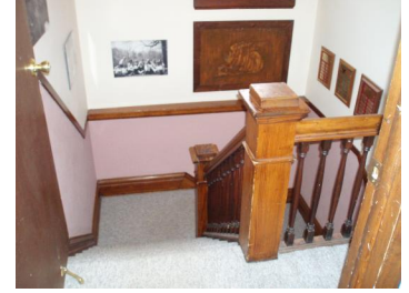
Stairway is the only access to the second floor. Prevents use by all people.
